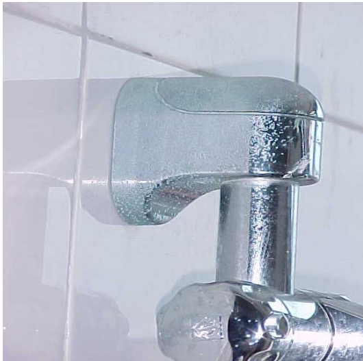
Corroded Shower Head Holder from Chlorine vapour
